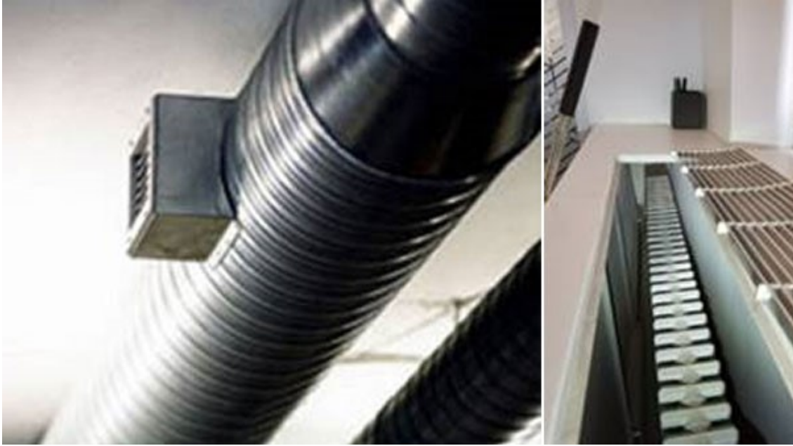
Air ducts and heating vents can allow sound to pass freely between rooms
