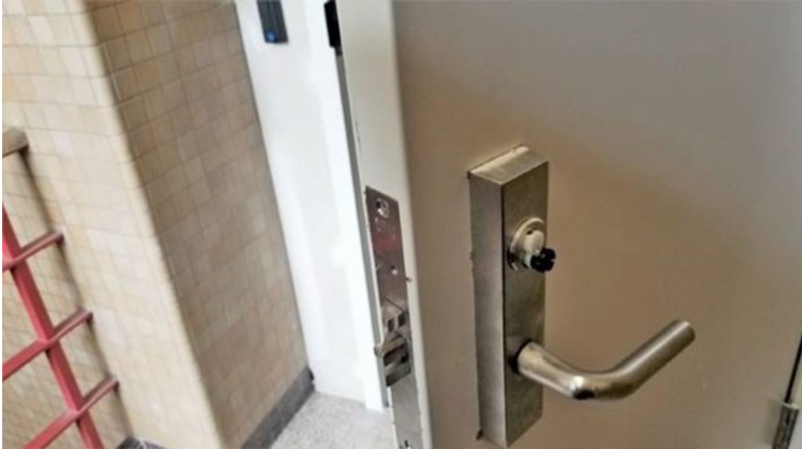
Damaged fire stair door allowed access to secure area with use of a coin.
